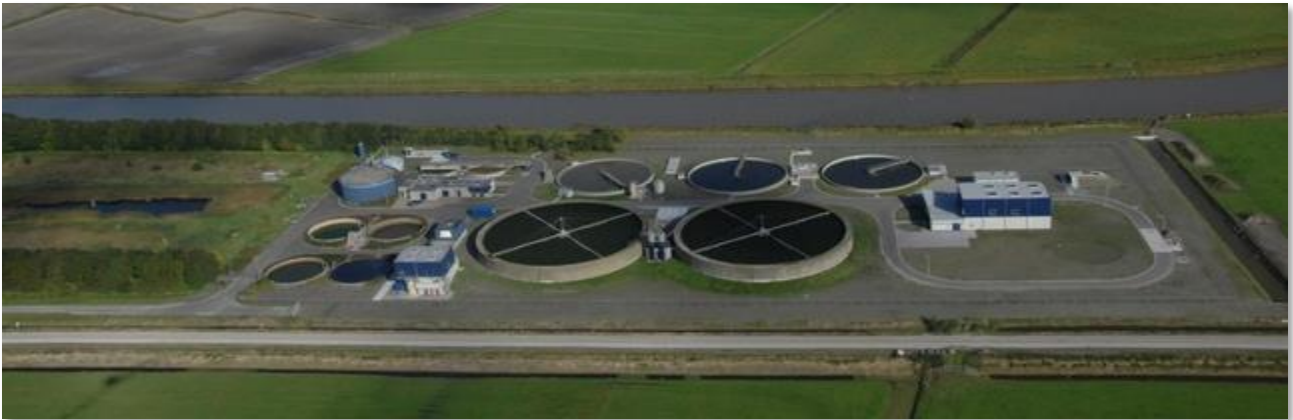
Figure 2 – Birdseye view of WwTW Franeker (site 1) with the MBF plant on the right
