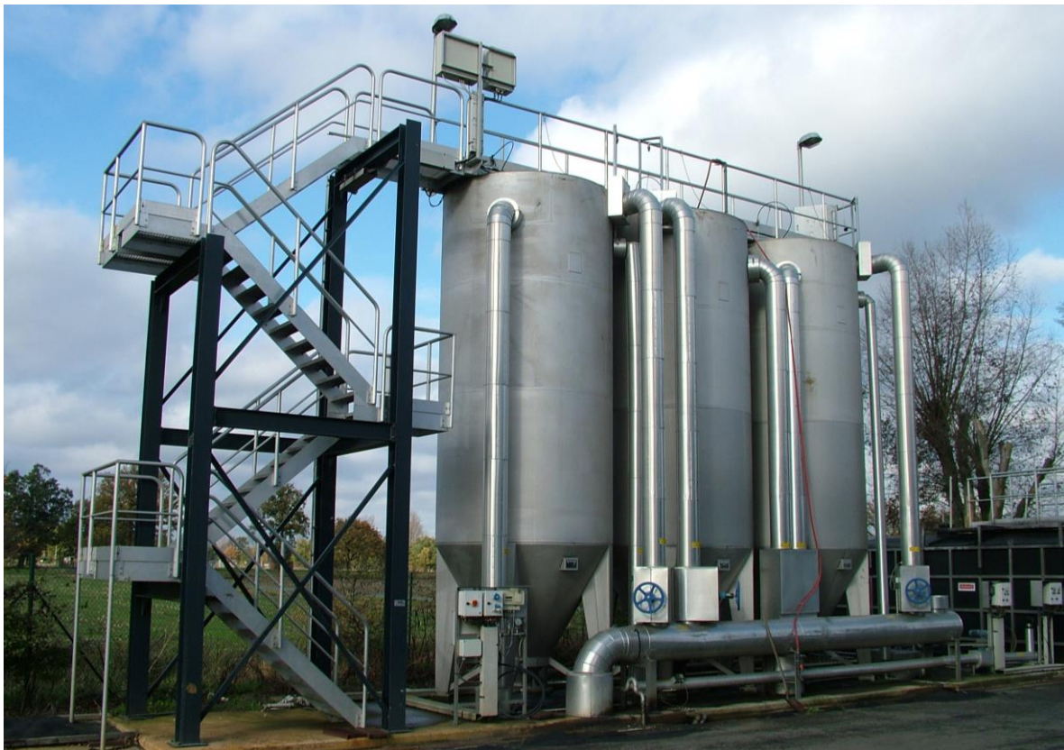
WwTW Bree tertiary denitrifying DynaSand filters
